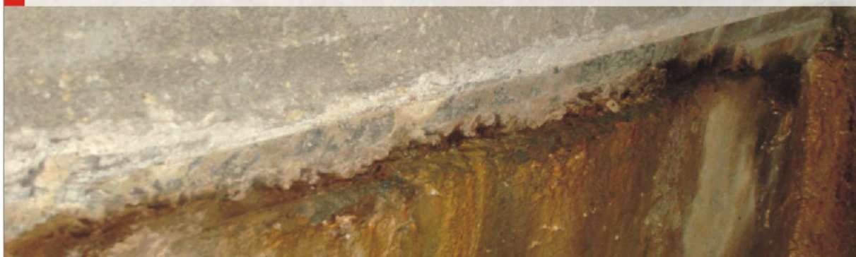
Leakage construction joint / Mạch ngừng thấm nước
